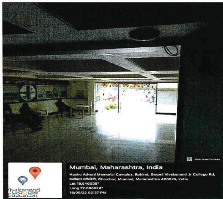
Wi-fi Router at Ground Floor
