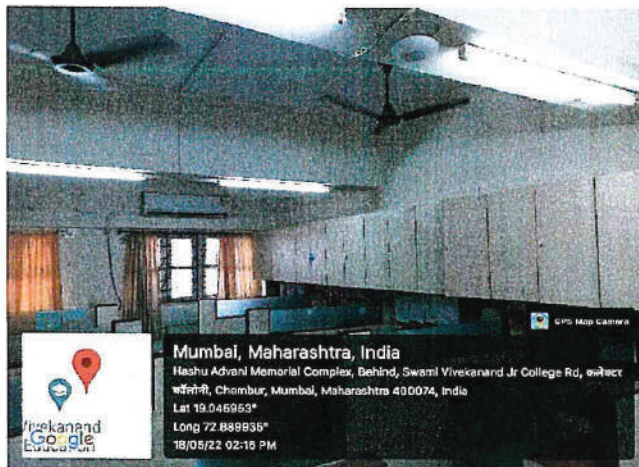
Wi-fi Router at Sixth Floor Faculty Room
