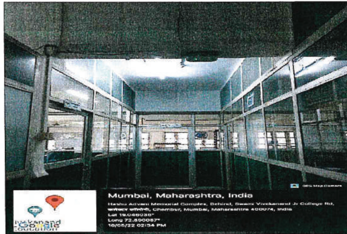
Wi-fi Router at First Floor corridor
