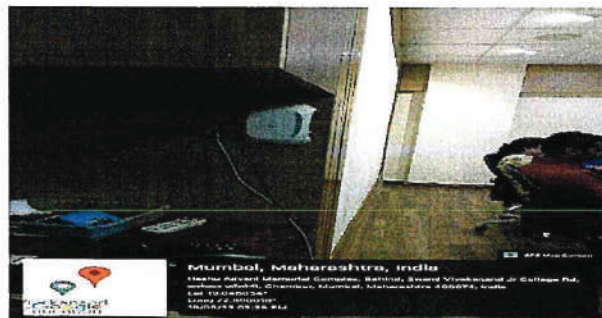
Wi-fi Router at Second Floor Board Room
