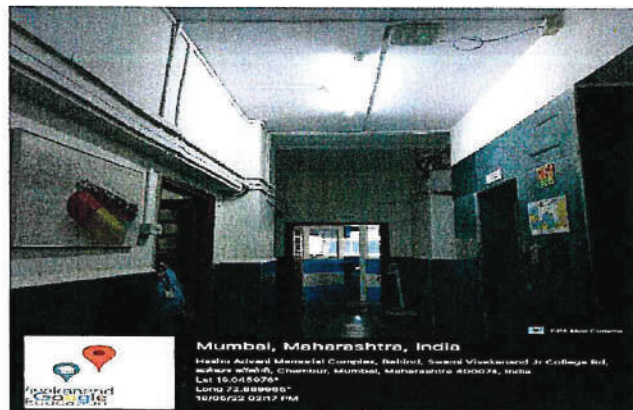
Wi-fi Router at Sixth Floor corridor
