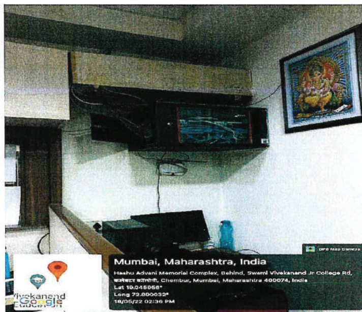
Wi-fi Router at Office Ground Floor
