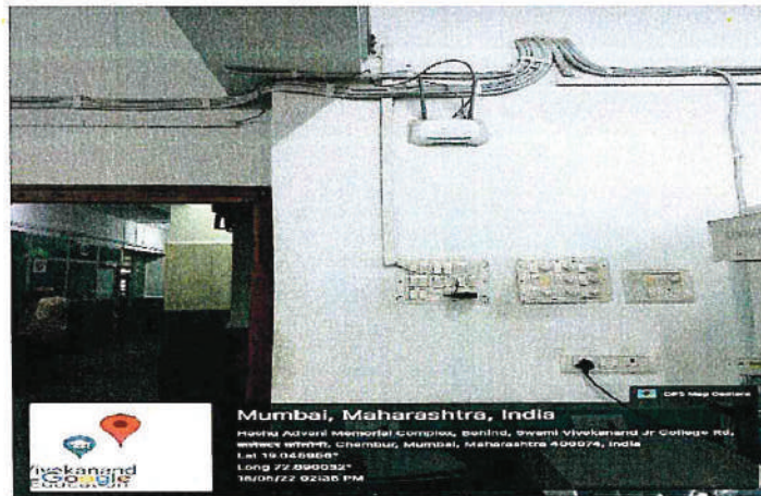
Wi-fi Router at First Floor Lab
